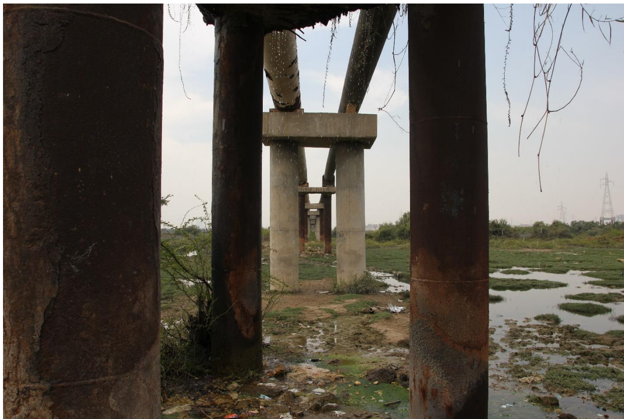
Rusted and leaking pipelines in Korangi industrial area, provide water to District west
